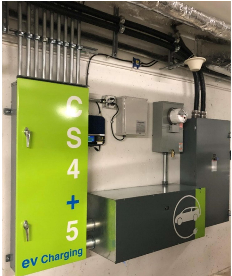
Figure 4: EV Ready Infrastructure in a multifamily building parking garage. Source: AES Engineering.
